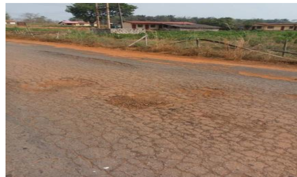
Figure 4: Failed portion of the road at Ufuma
