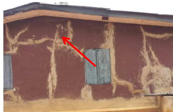
Figure 2: Patched cracks on the wall due to expansive soil at Ugwuoba
