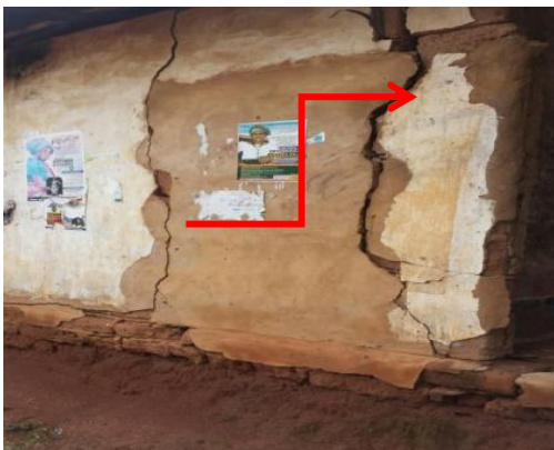
Figure 1: Abandoned building due to cracks at Ugwuoba
