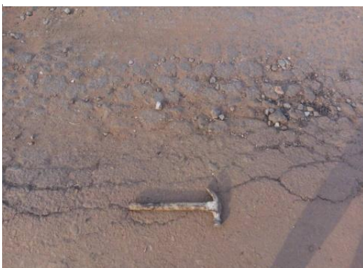
Figure 3: Failed Portion of the road at Enugwu-Agidi
