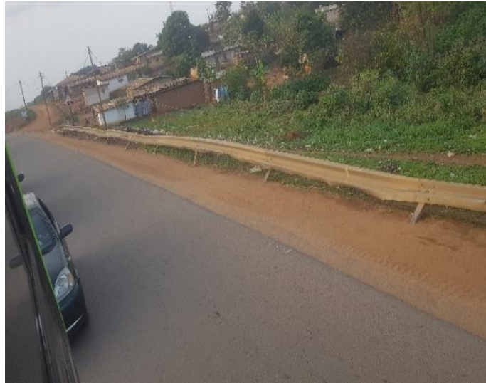
Figure 4. Guardrails in bad condition
