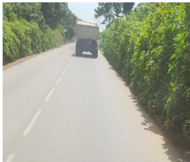
Figure 3. shoulders overgrown by weeds
