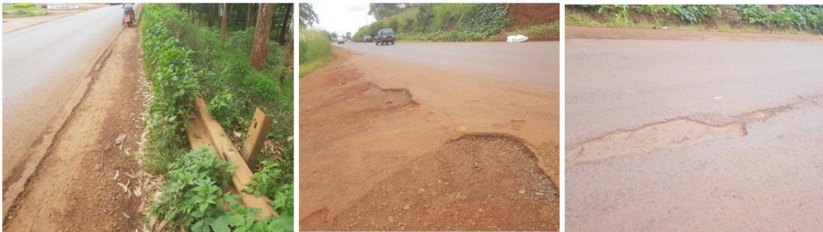
Figure 5. State of road surface
